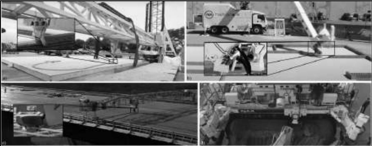
Figure 5 – 3D-Printer based technologies in construction a) – concrete additive manufacturing [8]; b) – bricklaying additive manufacturing; c) –rebar tyer; d) – slipform paver [11]
