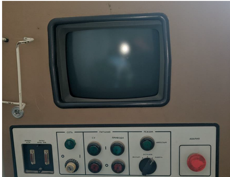
Fig. 1. General view of the control cabinet Puma Mark III (Sphere-36 (56))
